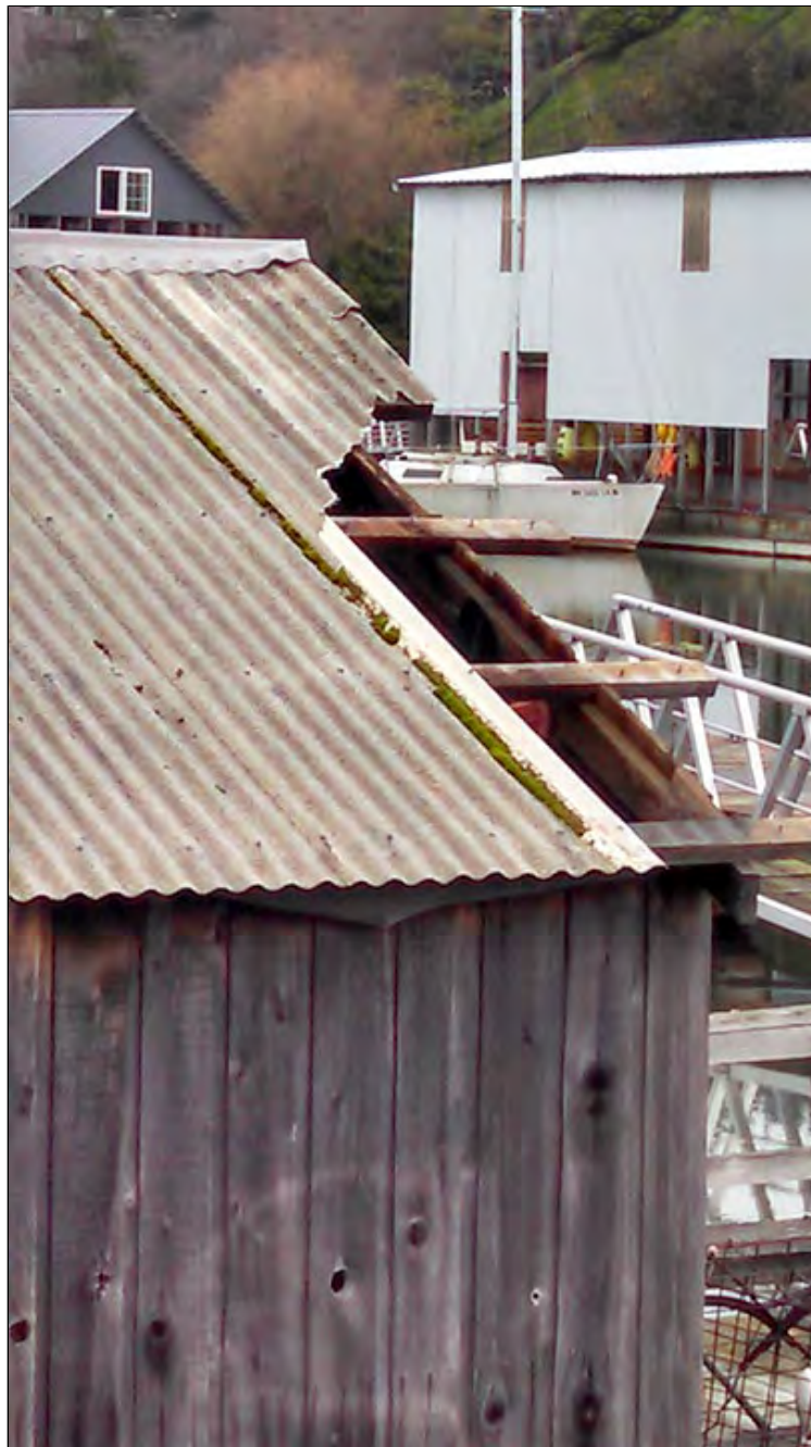
Figure 6.3 above A Sandy Hook, Whidbey Island, boat shed lost a portion of its roof during the high winds. Photo by Charlie Phillips.
